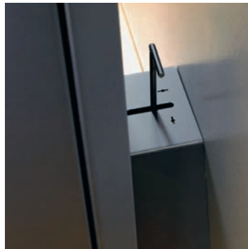
Shield and damper behind stove
